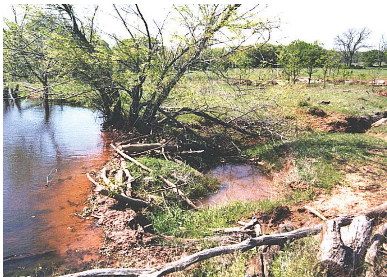
Livestock eroded trail and beaver dam located in the emergency spillway.
